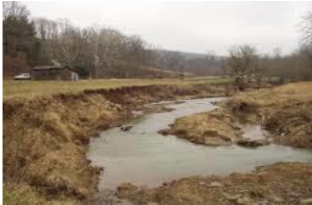
Figure 2.7 Stream Bank Erosion ( Source: http://www.dep.wv.gov )
