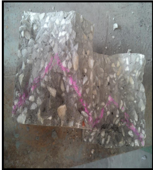
Fig.3.10 Depth of water penetration
