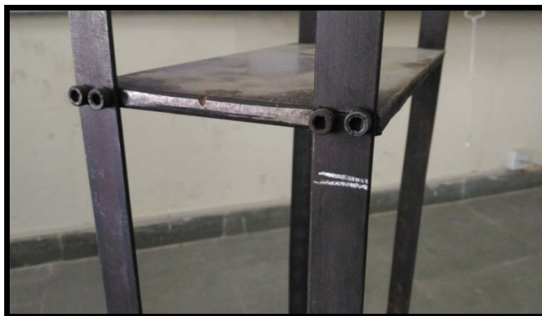
Figure.3.13:-Damage Structure 02 Refer (3.14B).
