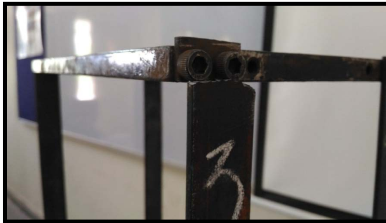
Figure.3.12:-Damage Structure 01 Refer (3.14A)
