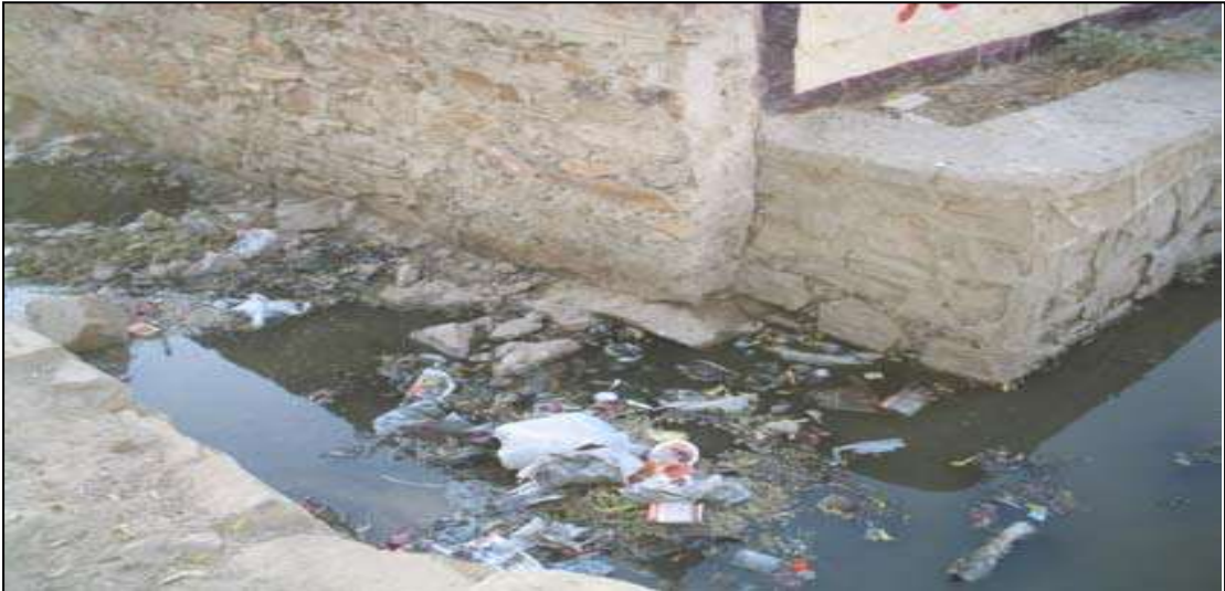
Photo 3.20: A Choked Minor Drain at G-Block Area, Mankarwali Road
