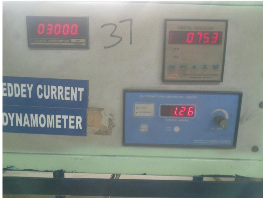
Fig. 3.2 Control panel of the eddy current dynamometer
