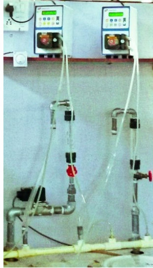
Figure 3.18: Dosing arrangement by using peristaltic pumps
