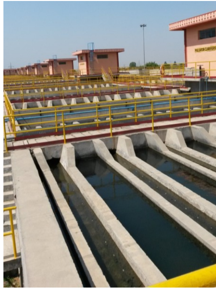
Figure 3.6: Series of Superpulsator ® units at the Surajpura WTP
