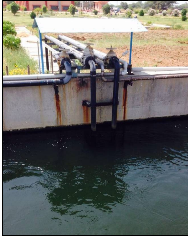
Figure 4.1: Pre-chlorination arrangement in raw water at Surajpura WTP
