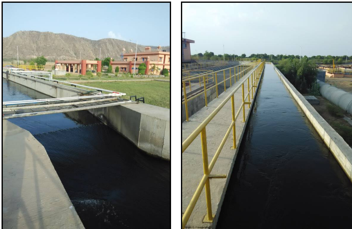
Figure 3.4: Surajpura WTP Pictures showing the (i) PAC dosing just before the Parshal Flume and (ii) Long Clarifier Feeding Channel
