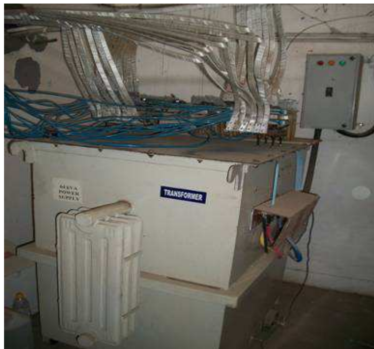
Figure 3.6. Photograph of 64 kVA Transformer.
