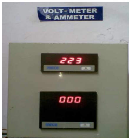
Figure 3.11. Photograph of Ammeter and Voltmeter.
