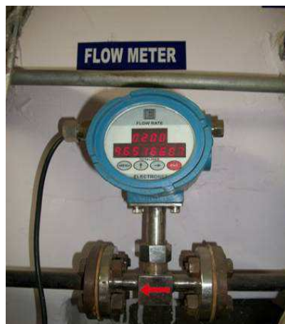
Figure 3.9. Photograph of turbine type flow meter.
