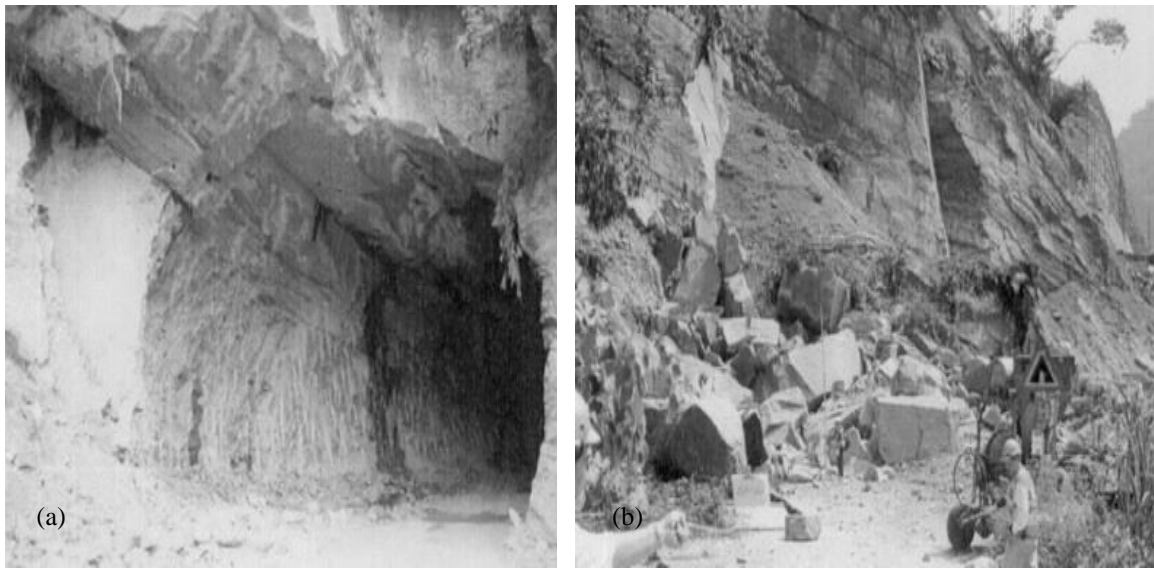
Fig. 2.4. Damage to Ching-Shue tunnel. (a) Tunnel entrance before the Chi-Chi earthquake; (b) Closure and damage of tunnel entrance due to slope instability (Wang et al. 2001)
