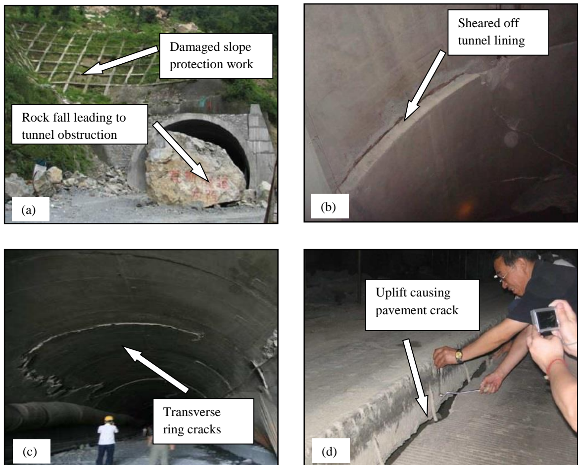
Fig. 2.5. Damages at Longxi tunnel during 2008 Wenchuan earthquake (Modified after Tao et al. 2011): (a) Rockfall obstructing tunnel entrance; (b) Sheared off tunnel lining; (c) Transverse ring cracks; (d) Pavement cracks due to uplift
