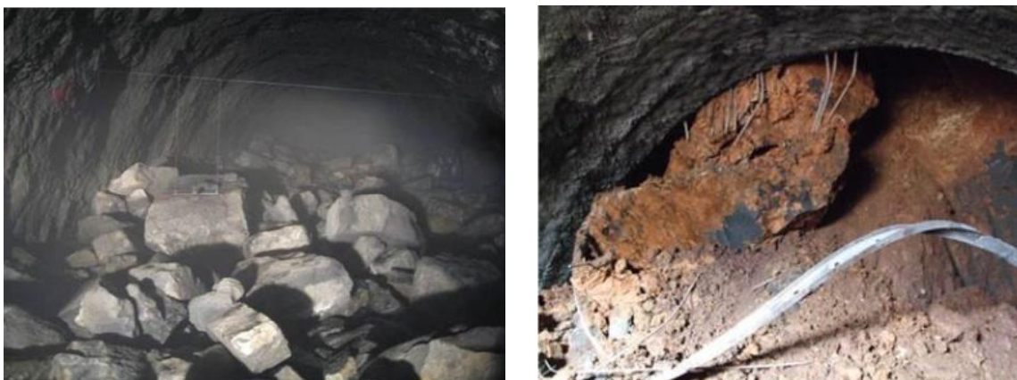
Fig. 1.1. Cases of instabilities during excavation (a) detachment of rock blocks and (b) collapse of the opening ( Zhu et al. 2017)
