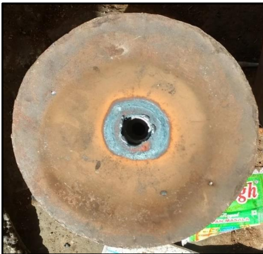
Figure 3.19: Inside view of the header
