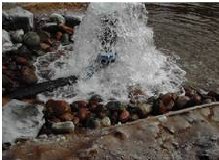
Figure 2.12 : Major Leakages (Bursts)
