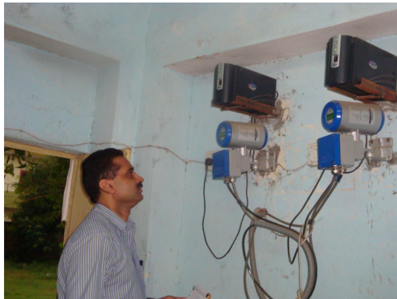
Photograph 5.1: Bulk Meter Reading at Malaviya Nagar Sector-9
