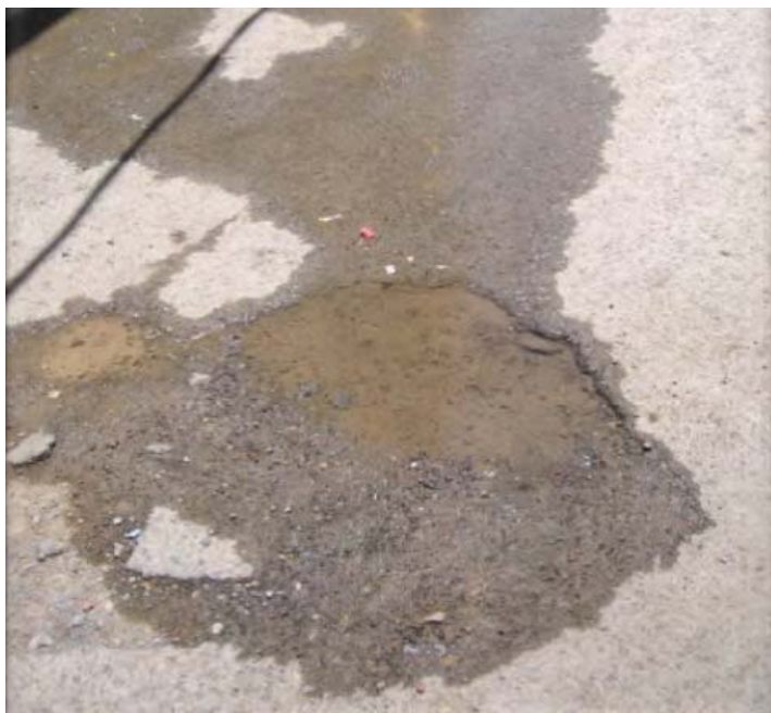
Figure 2.9: Leakages Visible During Supply Hours
