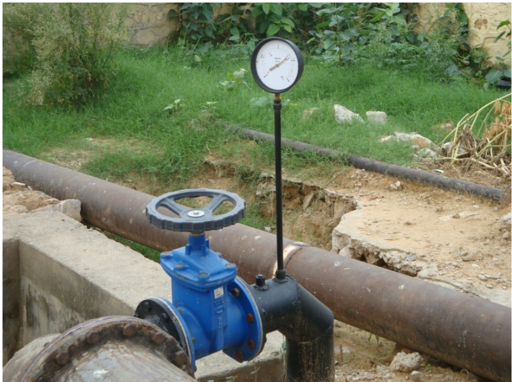
Photograph 5.6: Soft Seated Valve and Pressure Gauge at Malaviya Nagar Sector-9
