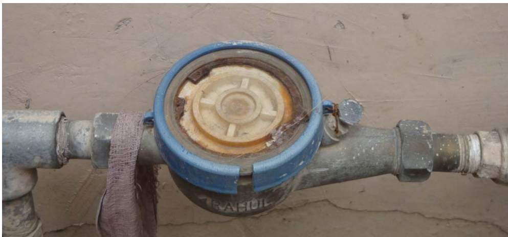
Figure 2.11: Non Working Water Meters
