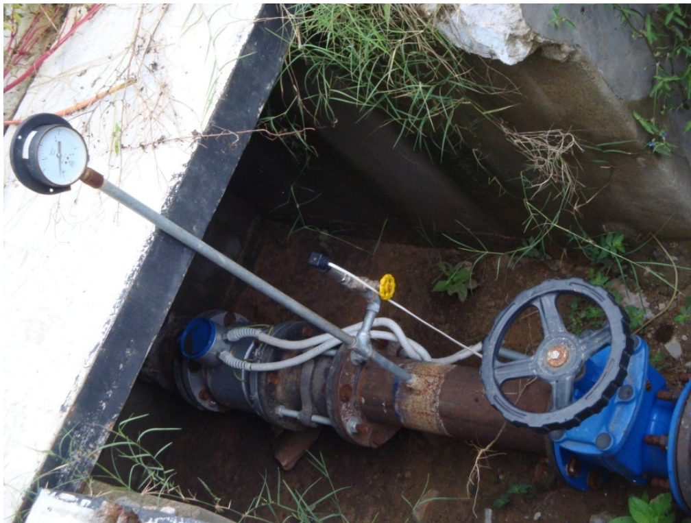
Photograph 5.4: Soft Seated Valve and Pressure Gauge at Masarovar Sector-3
