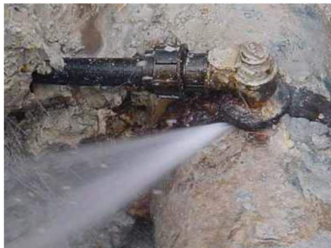
Figure 2.2: Leakages in Distribution Network [Farley, 2008]
