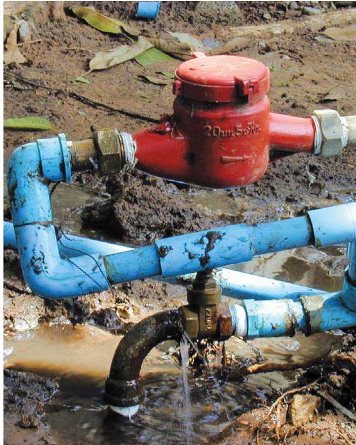
Figure 2.13 : Leakages on Service Connection
