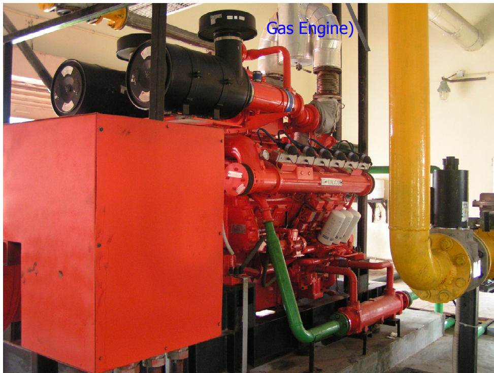
Figure 3.4 Biogas based power generation unit of STP Delawas Jaipur
