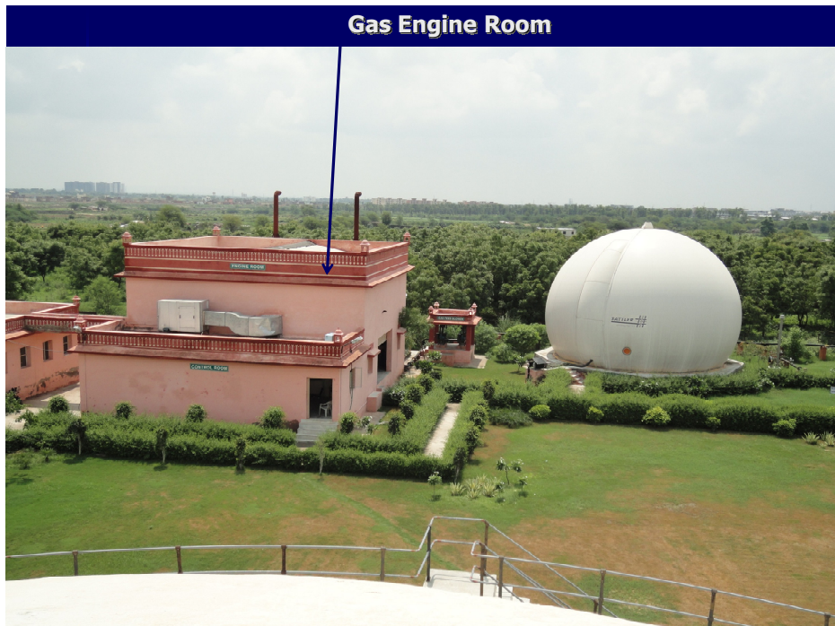
Figure 3.5 Gas holder and power generator room of STP Delawas Jaipur
