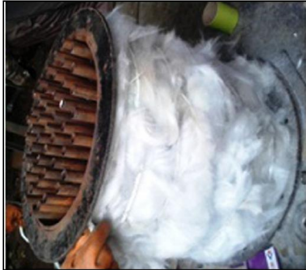
Figure 3.3: HRU with insulation of glasswool
