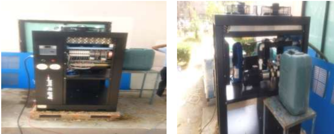
Figure 5-7: Chiller commissioning and testing
