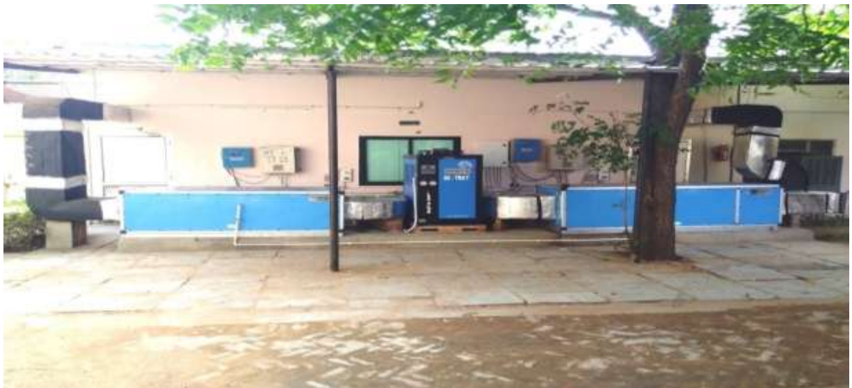
Figure 5-9: AHU of indoor-outdoor chamber after commissioning
