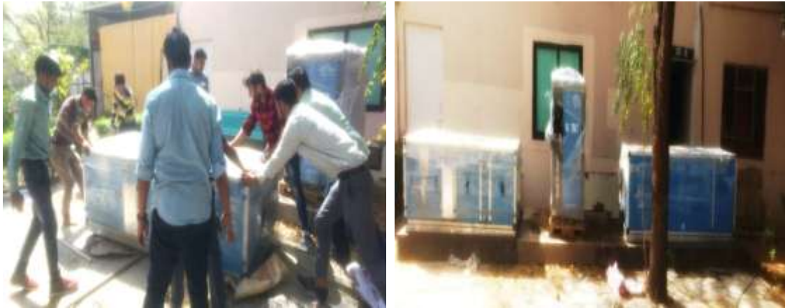
Figure 5-8: AHU commissioning for indoor-outdoor chamber
