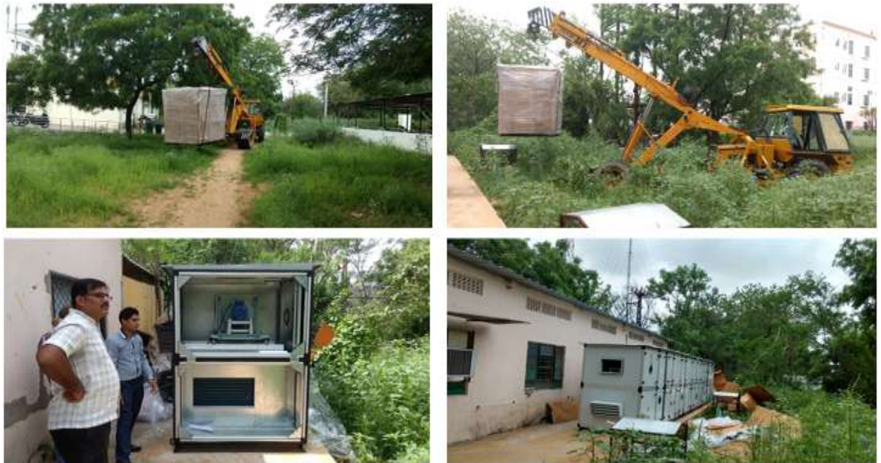
Figure 5-3: Installation and commissioning of modular DOAS
