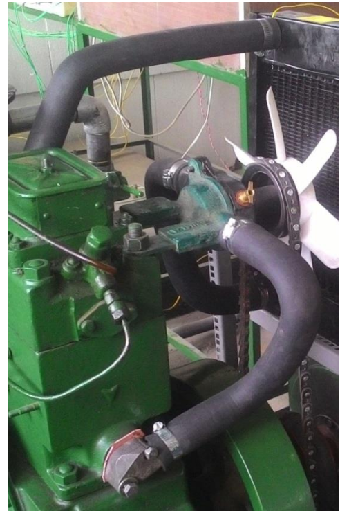
Figure 14: water manifolds and hoses
