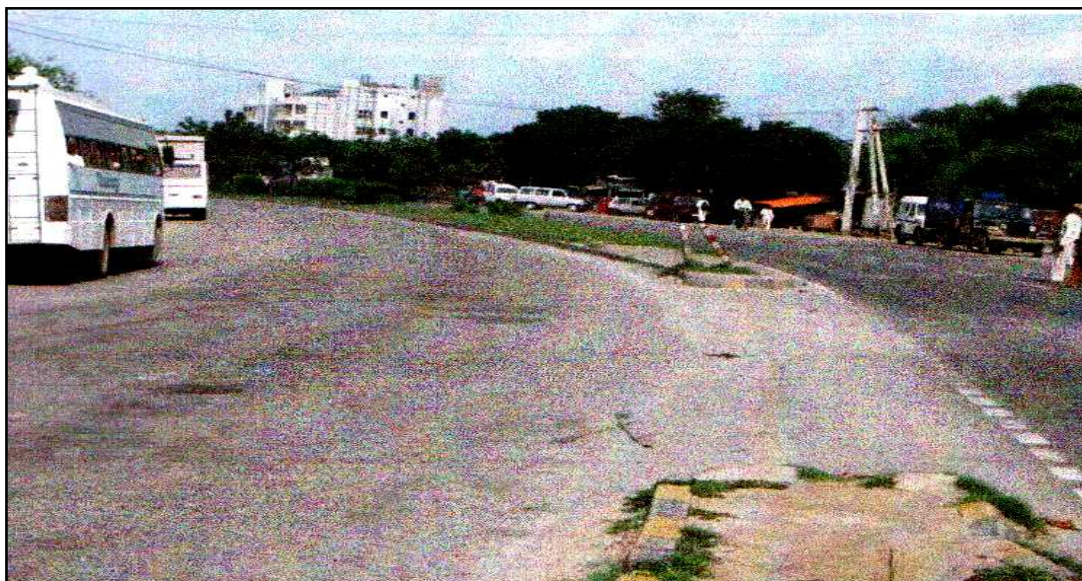
Photo 2. Poor Drainage due to Surface Water near Curves and Medians on NH-8
