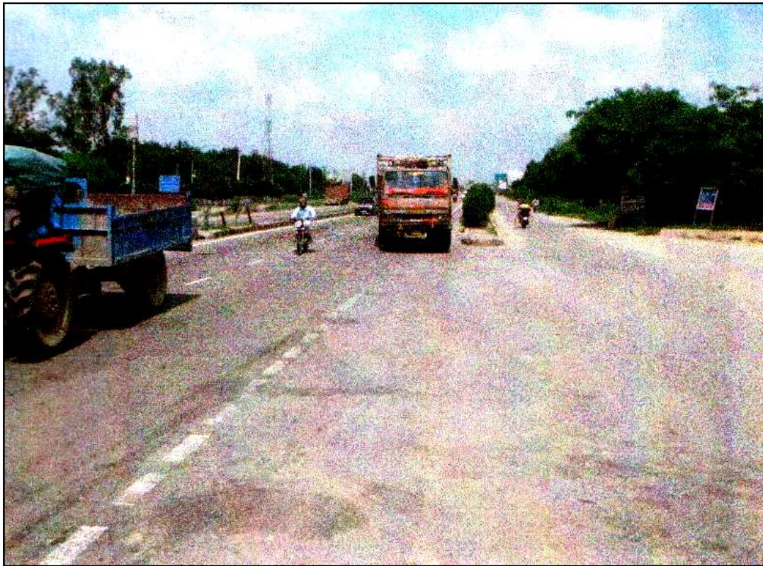
Photo 4. Poor Drainage due to More Water Retention Time on NH-8
