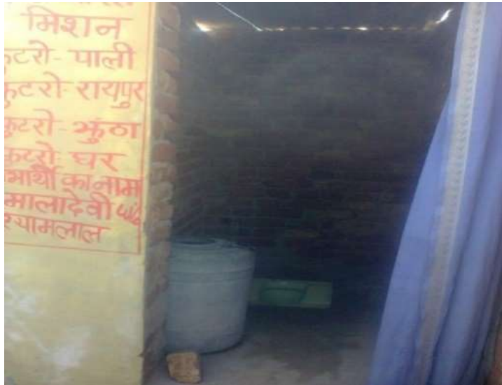
Figure 4.23: HH toilet in use at Jhoontha
