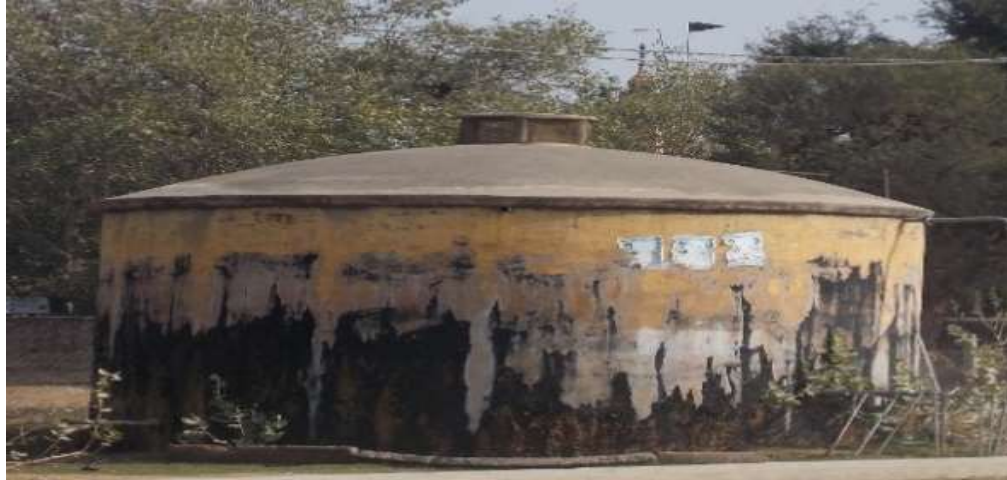
Figure 4.17: Clear Water Tank at Mohanbari
