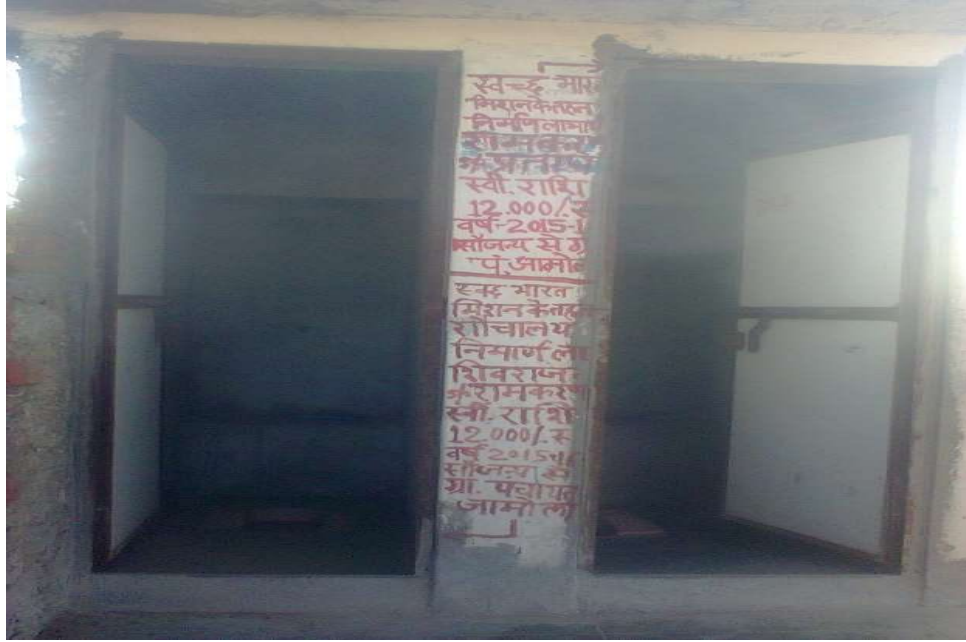
Figure 4.2: Household Toilets built under Swachh Bharat Mission in use
