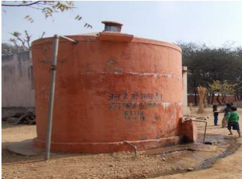
Figure 4.18: School Water Tank at Mohanbari
