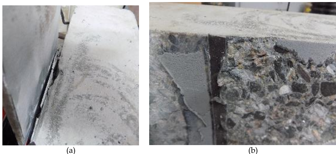
Fig. 6-9: Bearing zone failure in concrete specimen at interface for one mm thick adhesive layer; (a) crack lines at bearing end of interface after failure and (b) diagonally propagated shear crack in concrete specimen
