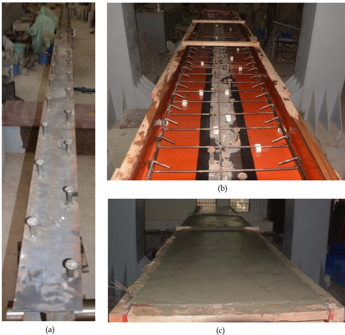
Fig. 7-11: Steel-concrete composite beam; (a) mechanical headed studs welded over steel beam in staggered pattern, (b) Prepared steel beam for concrete pouring along with reinforcement arrangement and (c) in place cast concrete slab
