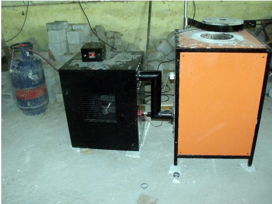
Figure 4.14 Details of Gas Fired Furnace
