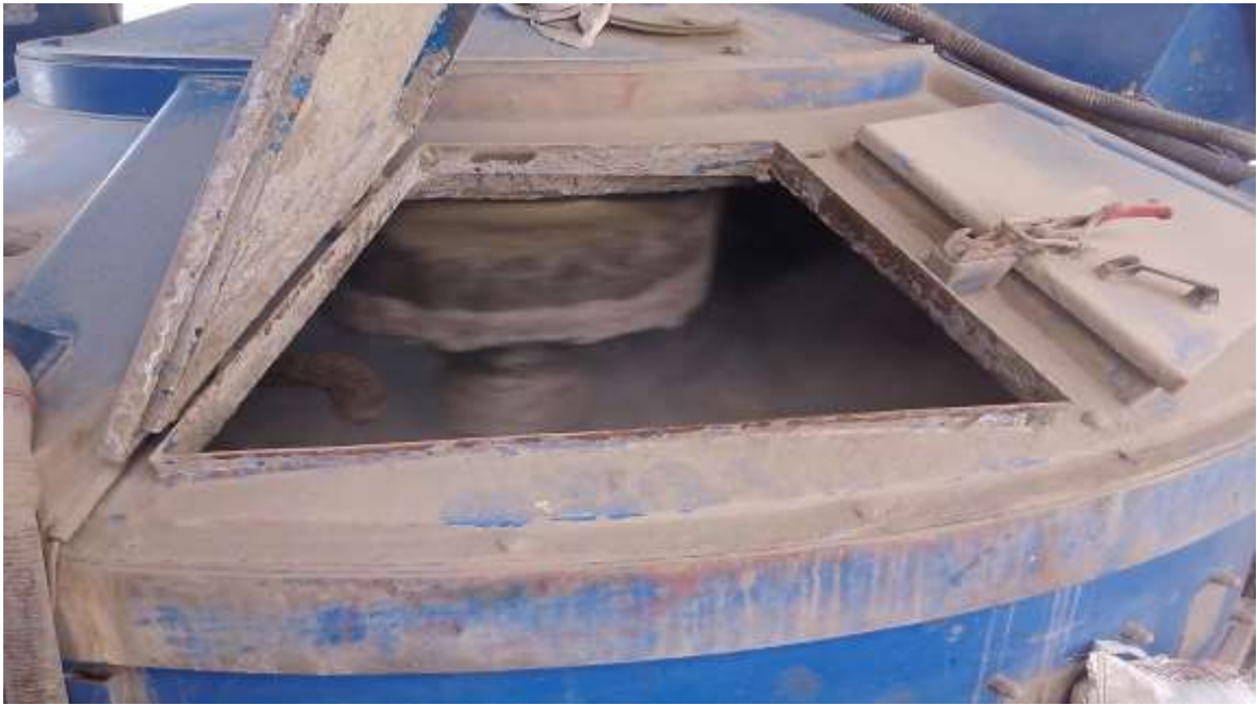
Picture 5: mixture machine at Pavcon
