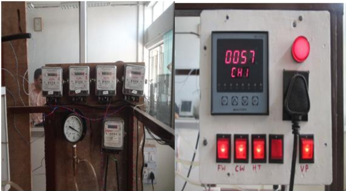
(f) Energy meters
