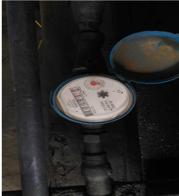
Figure 3.17 cooling water flow rate measurement
